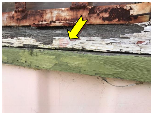
Photo 6. Exterior, throughout, window frames – suspected lead-containing white upper paint system.
