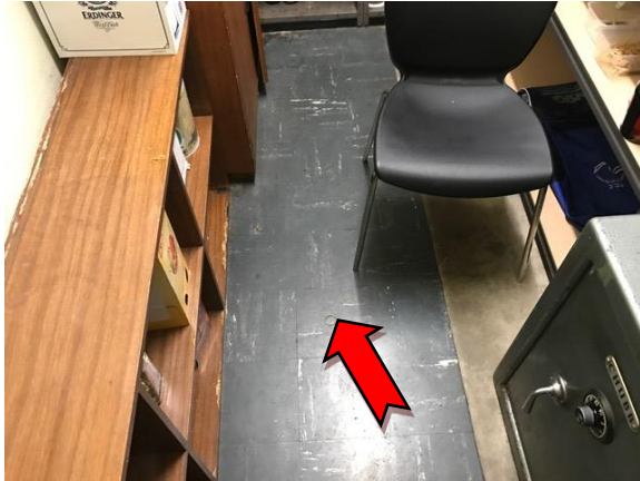
Photo 1. Interior, ground level, strong room, green floor covering – asbestos-containing vinyl floor tile.
