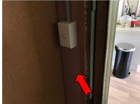
Photo 2. Interior, ground level, club room, wall lining – assumed asbestos-containing fibre cement sheeting
